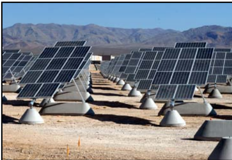
Nellis Solar Power Plant Clark County, NV
